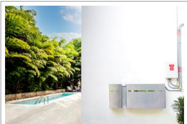
Cutler Bay Solar Solutions, Florida's largest family-owned solar-plus-storage installation company and a Platinum tier member of the Enphase Installer Network, has deployed more than 1.5 MWh of Enphase Encharge™ storage systems.
