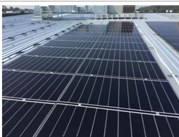
REA deployed an 80 kW solar system pairing its Power Series modules with Enphase microinverters for Innovative Stainless Steel in Brisbane, Queensland.
