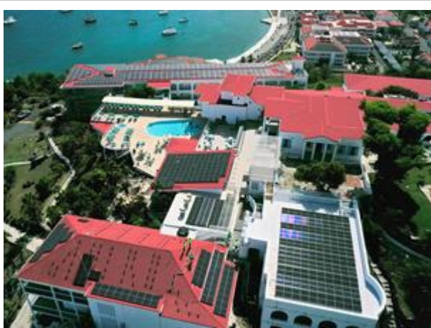
The commercial solar system installed by ProSolar Systems at Bluebeard's Castle Resort in the Caribbean, featuring Enphase microinverters.
